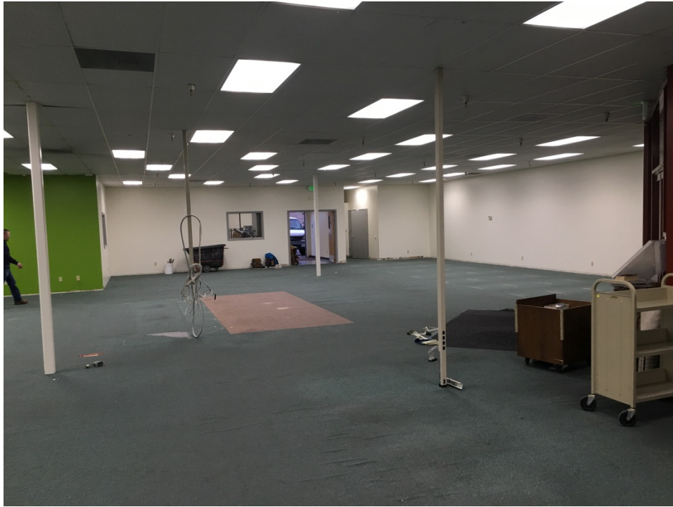
Old carpet at start of renovation – clearly shows the wear of use and time
